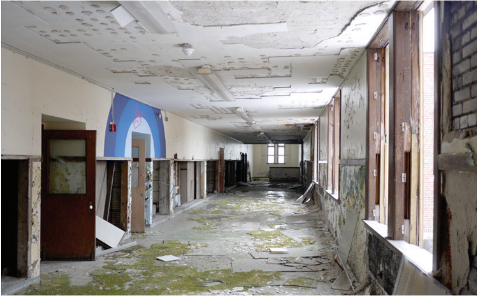
Water damage on the second floor has contributed to structural deterioration of the floor slab. The corridor floor slabs may need to be replaced.
