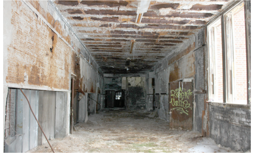
The first floor corridors are heavily water damaged and scrapped, with no original finishes intact.
