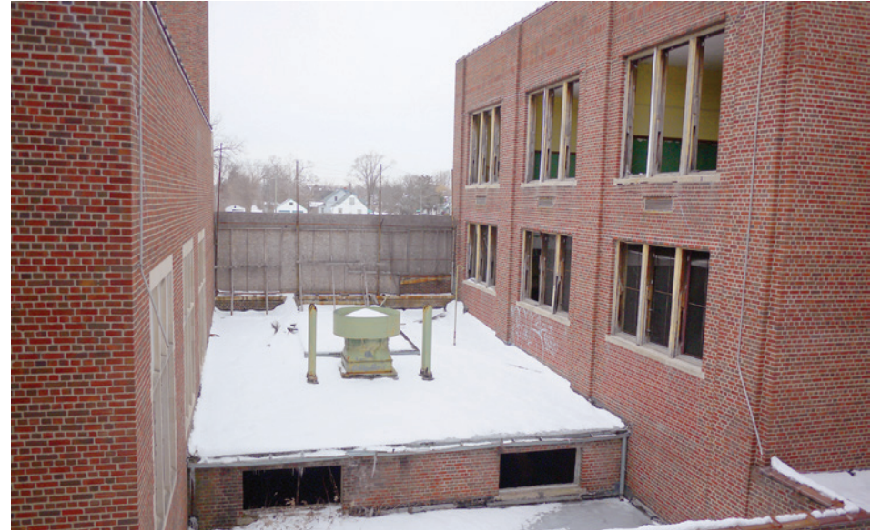
The central courtyard viewed from the second floor south corridor. The courtyard allows light and fresh air, but is not accessible from inside or outside the building, due to the raised boiler room roof.
