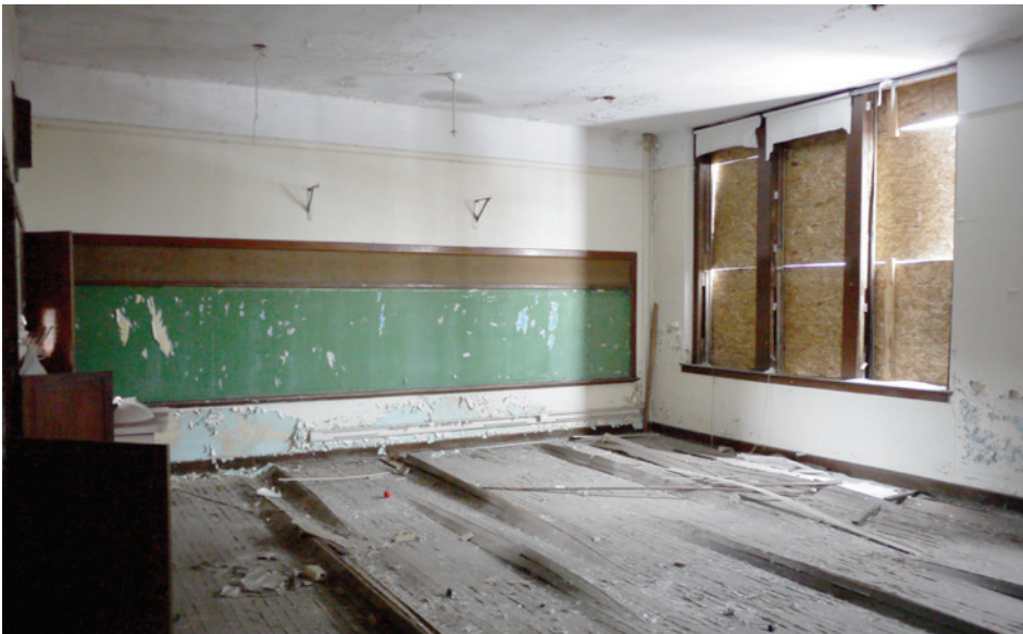
A typical classroom with plaster finishes in fair condition. The original wood-framed windows are missing throughout the school, and wood floors are buckled throughout.
