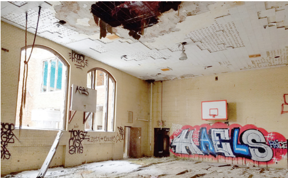
The gym is a mass-masonry brick box with tall arched windows. The wood roof deck has deteriorated, resulting in water damage to the ceiling and floors.
