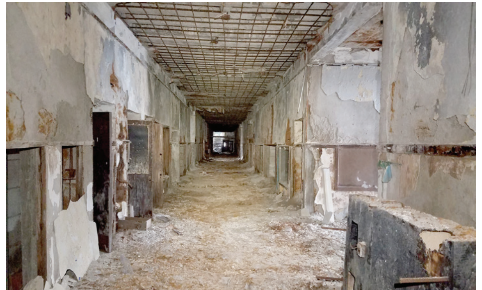
The interior has suffered from a great deal of water infiltration on both floors. The first floor main corridor shown above has had major deterioration of its plaster finishes; gypsum block non-bearing walls are also vulnerable to water.
