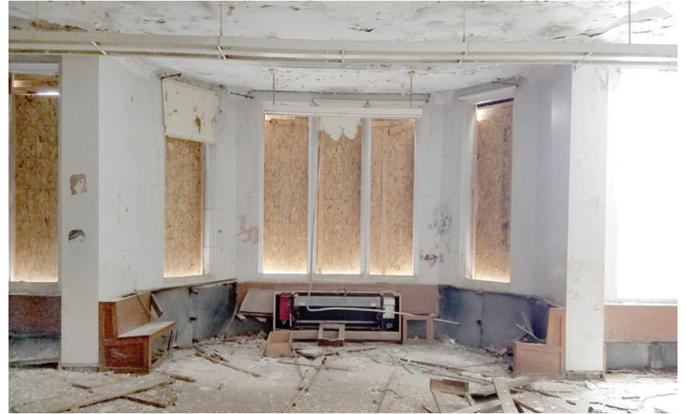
A special classroom (formerly "teacher rest") located on the second floor in the center of the main wing. This room and the library below both feature a bay window and fireplace.
