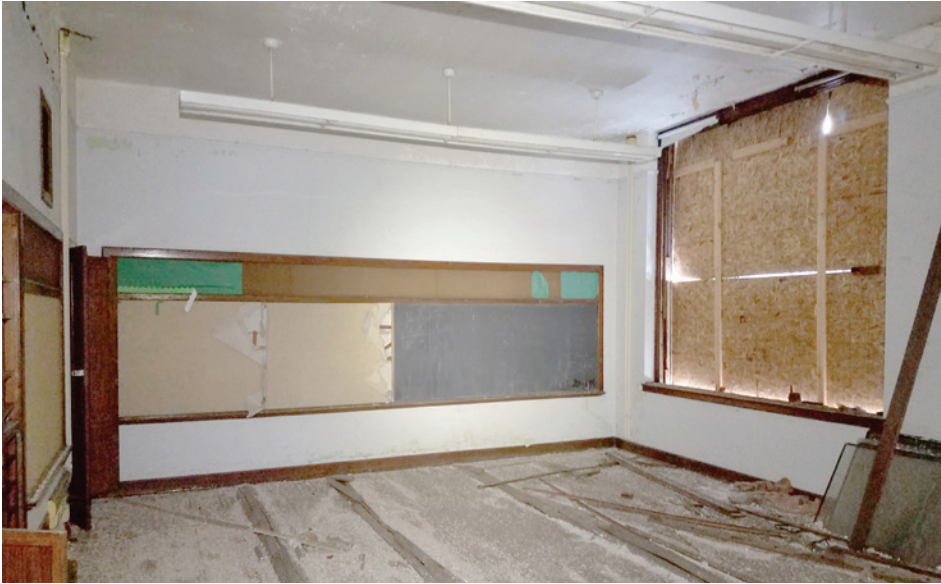
A typical classroom with finishes in good condition. Many other classrooms have suffered from water damage.
