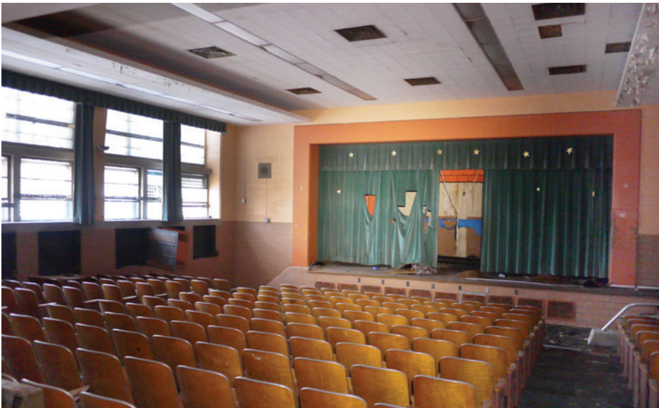
The simple concrete-block auditorium was built as part of the 1955 addition. It is in good condition, with seats and finishes intact.
