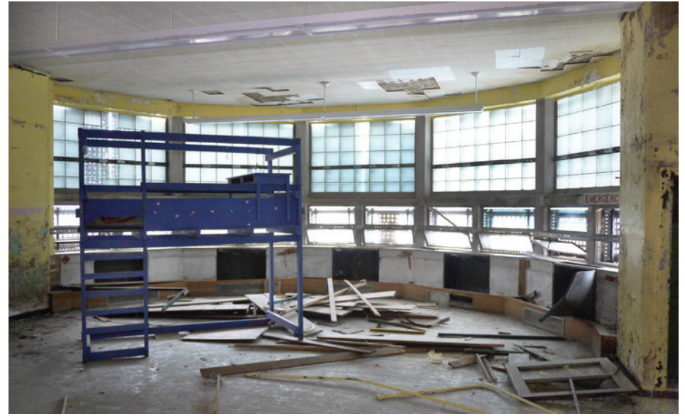
The kindergarten bay has a layout typical of schools from the 1920s. The windows were replaced with glass-block and operable steel-frame style to match the 1955 addition.
