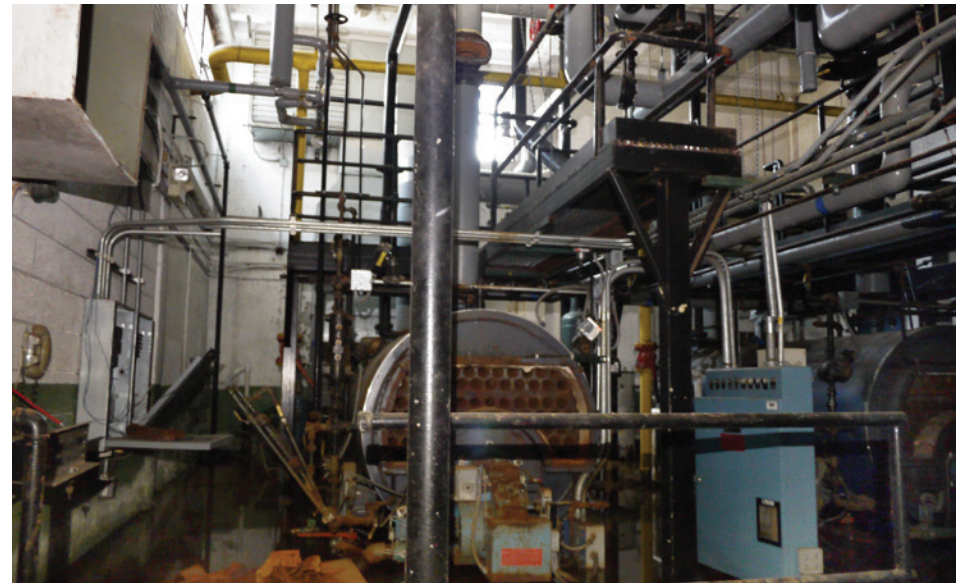
The school features an attached boiler room accessible from the main hallway. The space is a naturally-lit sunken cube, measuring almost 30 feet in all directions.
