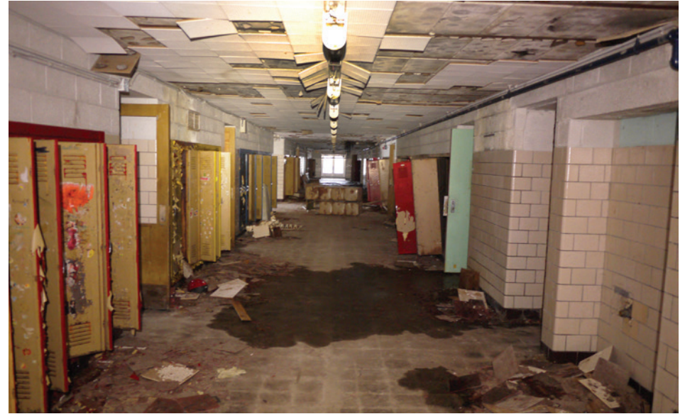
The main (north) corridor in the 1955 unit is 12' wide, but has only 8' ceilings—lower than at other historic schools. Water infiltration was observed throughout all corridors.
