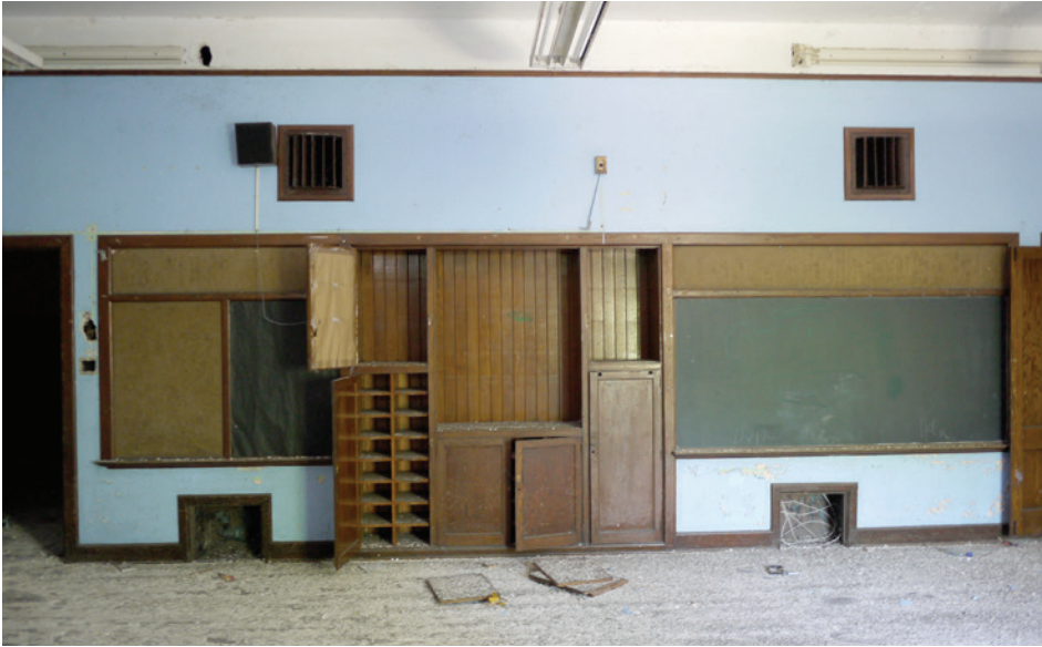
A typical classroom featuring built-in furniture and finishes in excellent condition. Although the school is open to trespass from the street, there is relatively little damage from vandalism, scrapping, and the elements.
