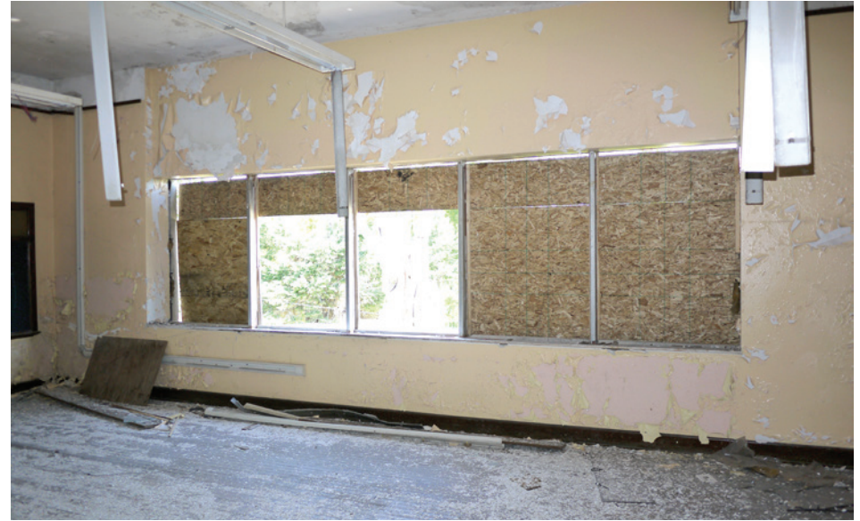
Classroom windows were partially filled in, leaving low strips instead of the usual tall openings seen in schools of the same era. The modern aluminum replacement frames have been scrapped throughout.
