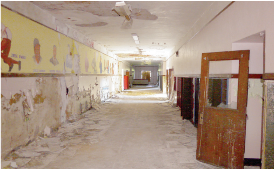
The north hallway on the second floor is single-loaded, with classrooms on the exterior side. Original windows overlooking the interior courtyard have been filled in. Hallways are painted with murals of civil rights heroes, celebrities, professions, and scenes from African and African American history.
