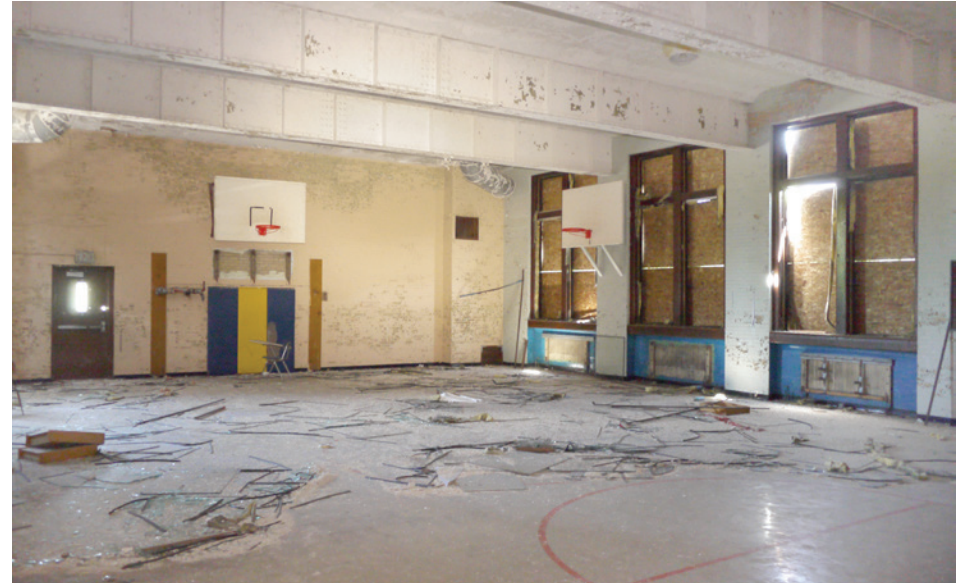
The gymnasium is in good shape, and appears to have been in use recently—debris has been swept away from beneath the basket. There does not appear to be water damage, and the floors have not bowed like most other gyms observed in this study.
