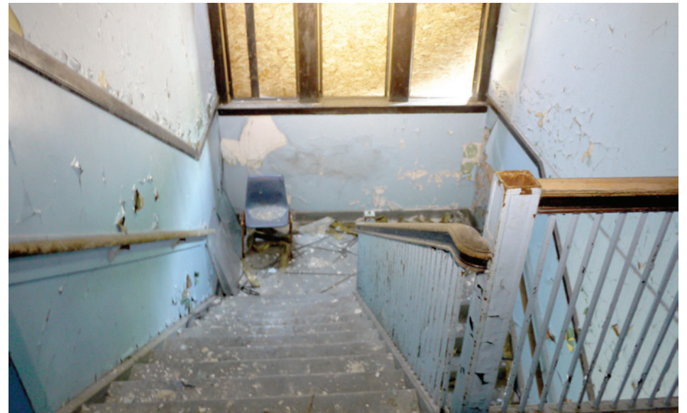
Stairwells in the original unit are tall and narrow; with flights of stairs at every entrance and a split-level first floor, this building is not ADA accessible.
