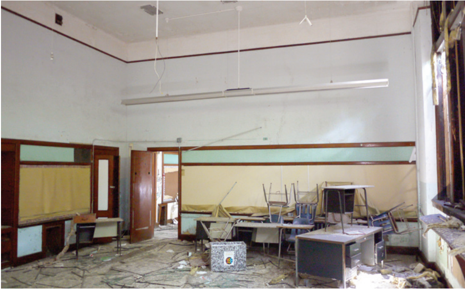
First floor classrooms in the 1923 (south) wing have 16-foot-tall ceilings, and high ceilings, giving the spaces a cavernous feel.
