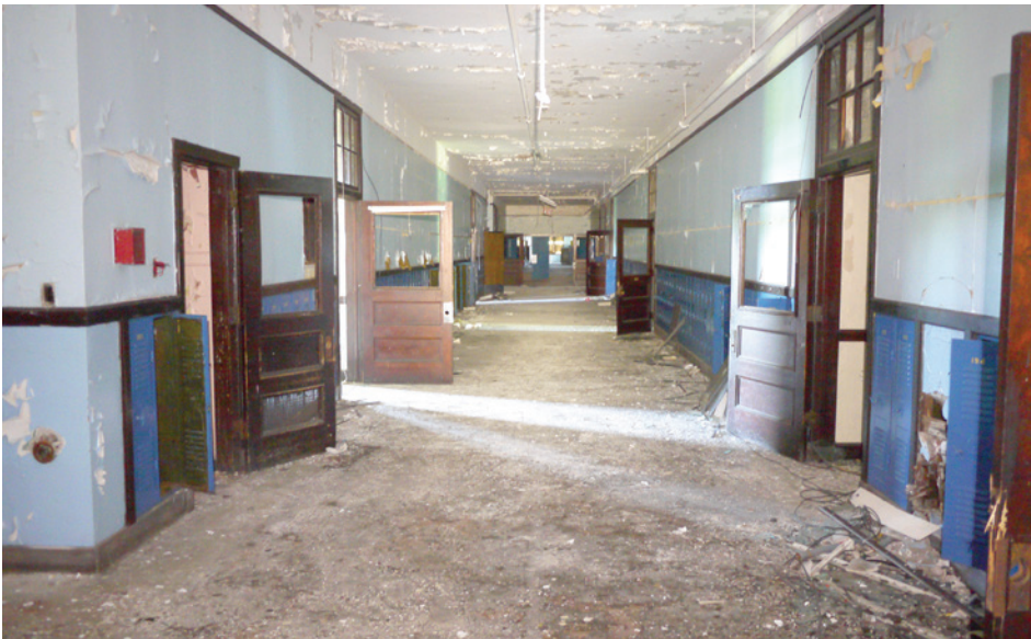
The first floor corridor of the 1923 unit, looking towards the 1916 unit. A short run of stairs is visible in the distance, where the two units join.
