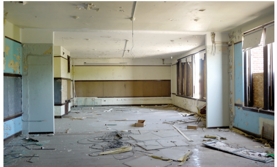
Two second-floor classrooms have been turned into one long room by removing the partition wall.
